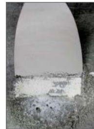
Blistered paint is easily scraped off in seconds!!!!
