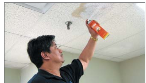
Stained ceiling tile
