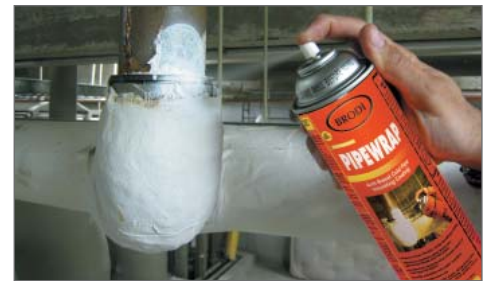
Copper pipe insulated with Pipewrap
